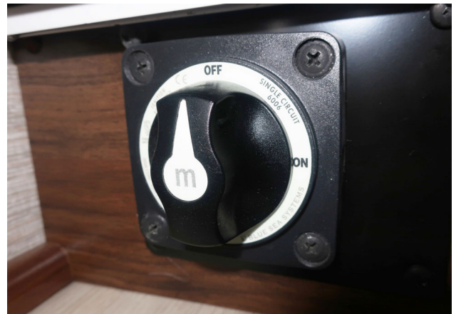
Inverter/charger disconnect switch. (Located inside entrance door next to awning controls -typical view)
